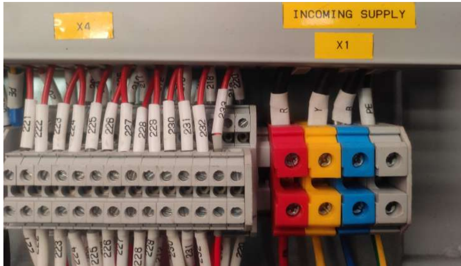
Figure 3-6 Electrical Connection - AC main line input at Control Panel
