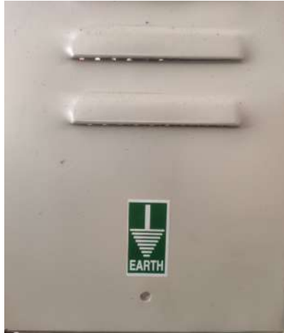
Figure 3-7 PE / Ground connection on Panel and Machine
