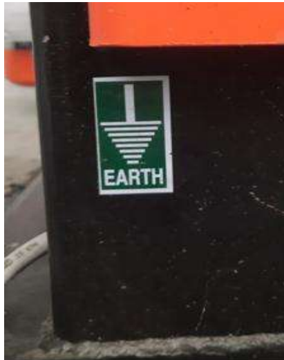
Figure3-6PE/Ground connection on Panel and Machine
