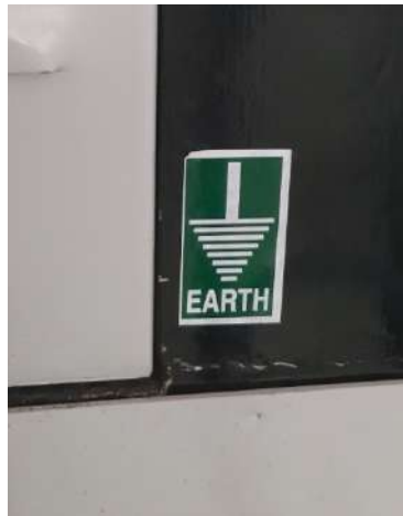
Figure 3-5 PE / Ground connection on Panel and Machine
